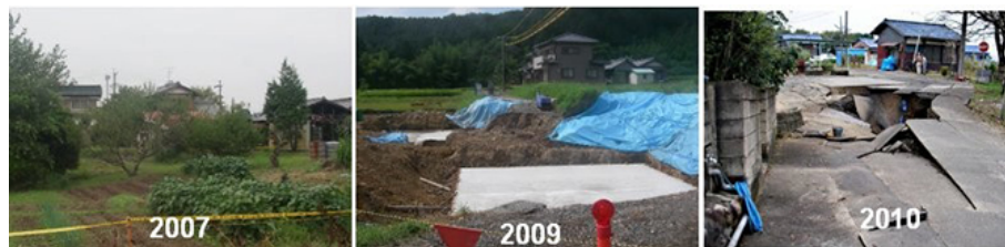
Figure 2. Large sinkholes occurred recently over the abandoned lignite mine in Mitake town.
