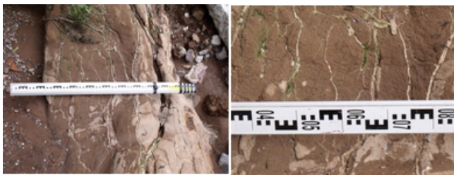
Figure 4. Filled cracks inside the zone of influence of the Oriente Fault. Refill consisted in groundwater caliche with a maximum thickness of 1 cm.
